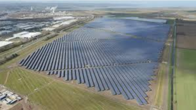
Solar park, UK
