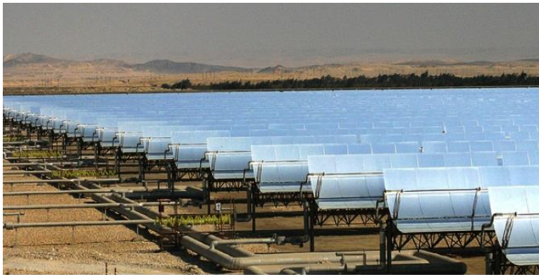
Parabolic trough, Egypt
